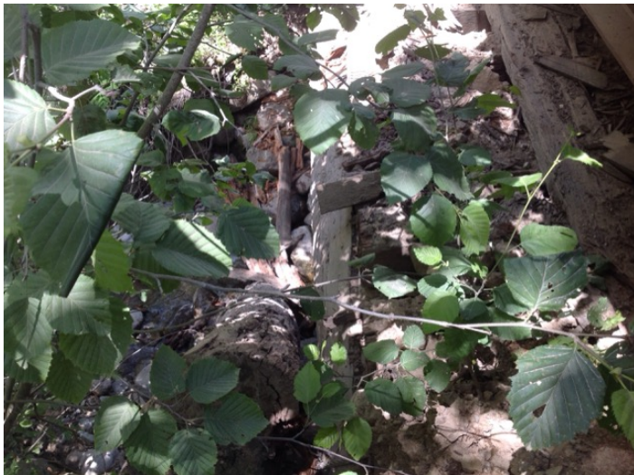
log stringer failure
