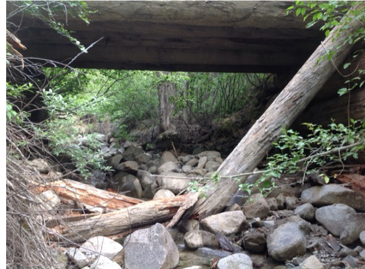
log stringer failure
